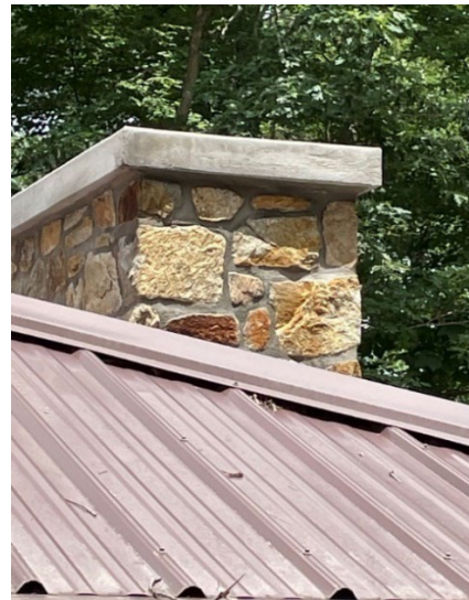
The chimney repair on the law enforcement cabin marks the final step in this building's renovation.
