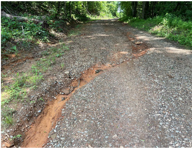
Erosion on Conservation Road creates potential impacts to visitor and vehicles.
