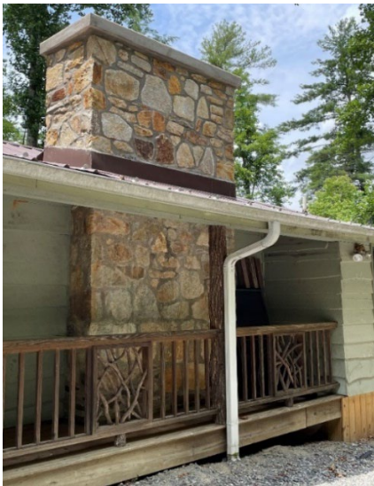
The chimney at the law enforcement cabin was repaired to eliminate leaks.
