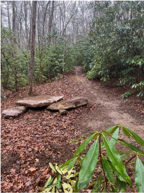
Removal of protruding rocks and repair of the trail surface to promote safety and sustainability of Grassy Creek Trail.
