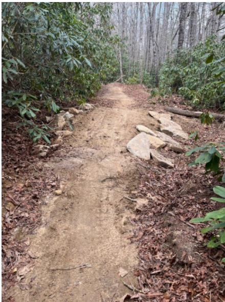
Construction of a turnpike along Grassy Creek Trail eliminates a chronically wet area and improves trail experience for visitors.
