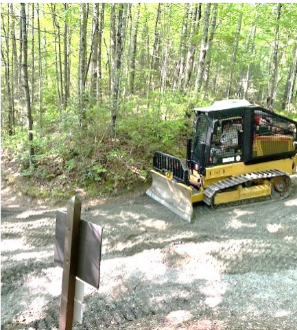
NCFS equipment operator reshapes the surface of the Triple Falls Trail prior to the gravel application.
